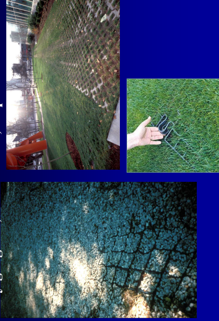
Temporary parking or access roads supported by geogrids, turf meshes, or paver blocks
