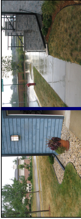
Disconnected roof drain
